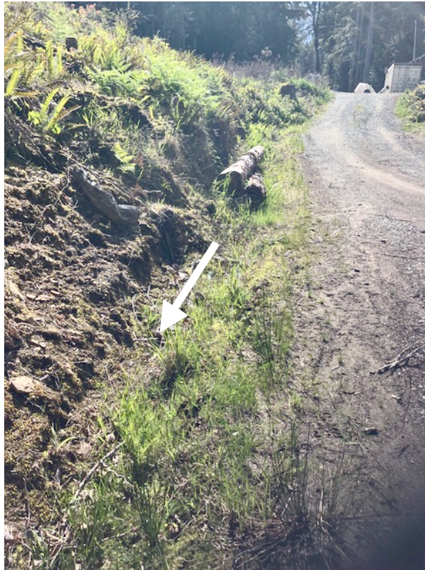
Photo 5. Drainage ditch along south side of roadway looking westerly along southern side of property, May 20, 2025. White arrow indicates drainage flow direction.
