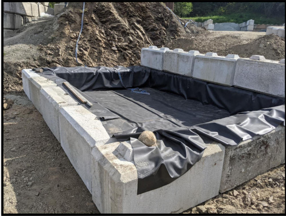
Photo 21 – Lined basin to capture overflow from batch plant water tank and as an area for the forming of concrete loc-blocs. Basin drains to batch plant water retention area.
