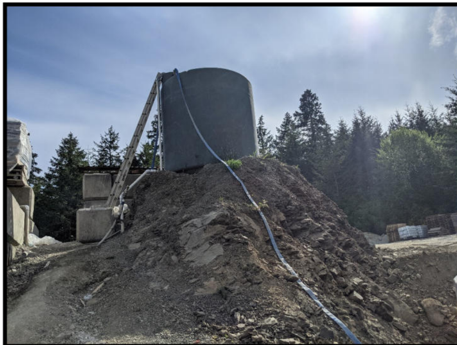
Photo 20 – Water tank used for concrete batching and overflow hose to newly constructed overflow basin / loc-bloc forming area.
