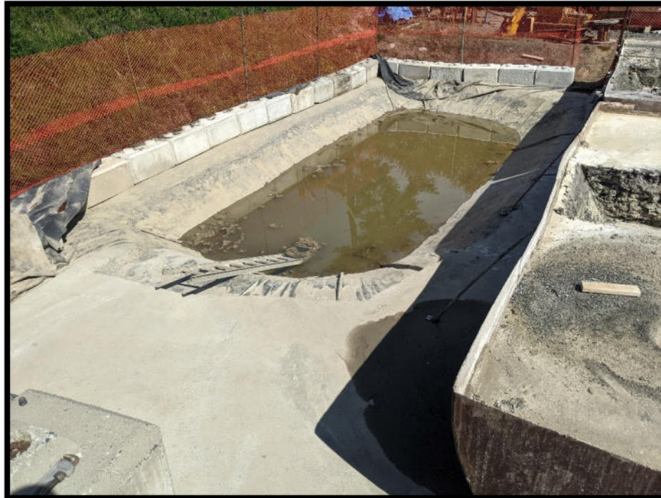
Photo 32 – Waste water retention area. Steel tanks were full of concrete solids at the time of inspection, so the lined secondary containment area, seen here, was in use to store waste waters.
