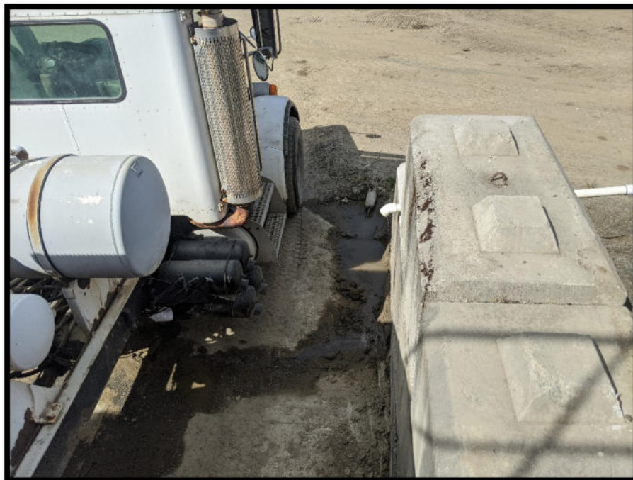
Photo 34 – Waters from within the batching area are directed to the waste water management area through this inlet.
