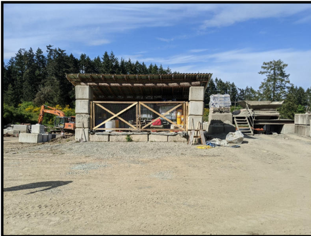
Photo 4 – Looking northeast at modified chemical storage shed, including new roof and lockable doors.
