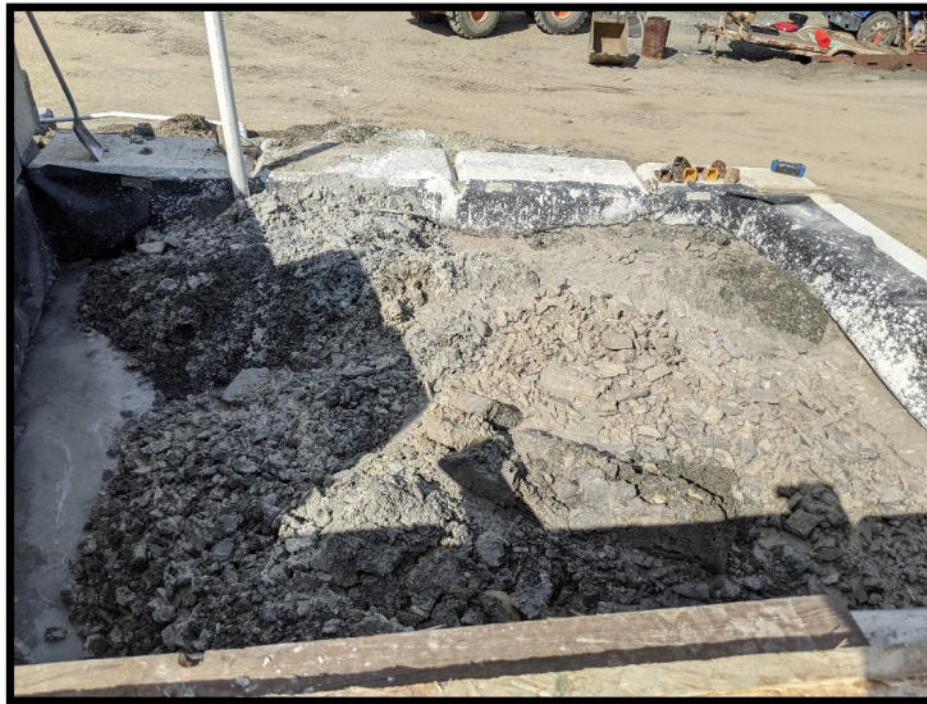
Photo 22 – Solids from concrete truck washout and plant cleaning are deposited within this lined basin to the east of the batching area where they can dry enough to be collected. Basin drains to batch plant water retention area.
