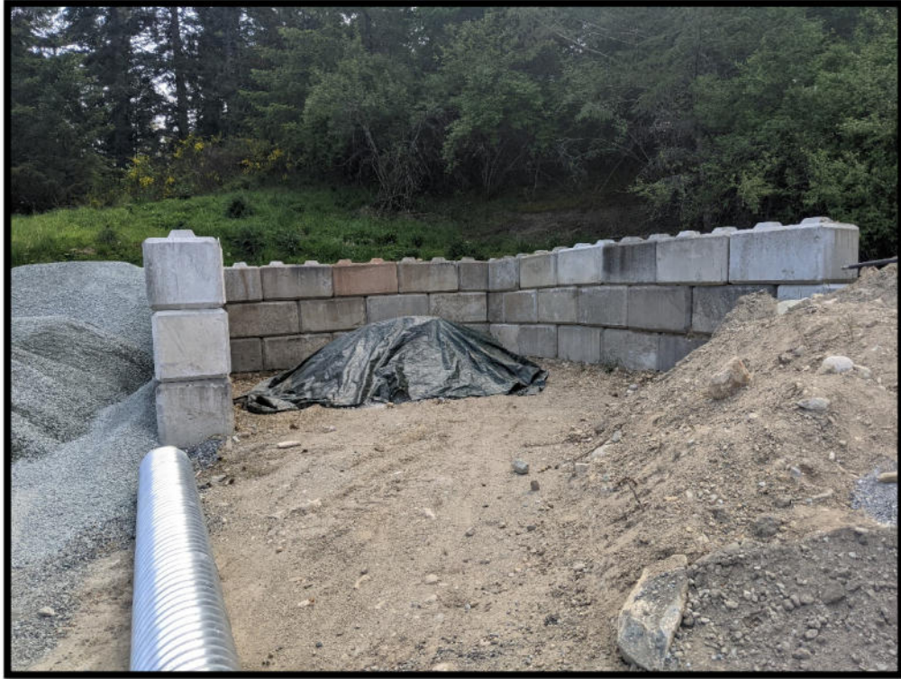
Photo 23 – Covered stockpile of excess concrete and dried sludge, to be re-used for loc-bloc production or as structural fill.
