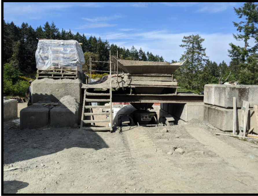
Photo 35 – View of batching area. Generally housekeeping could be improved to prevent dust and potential transport of sediments from the area.
