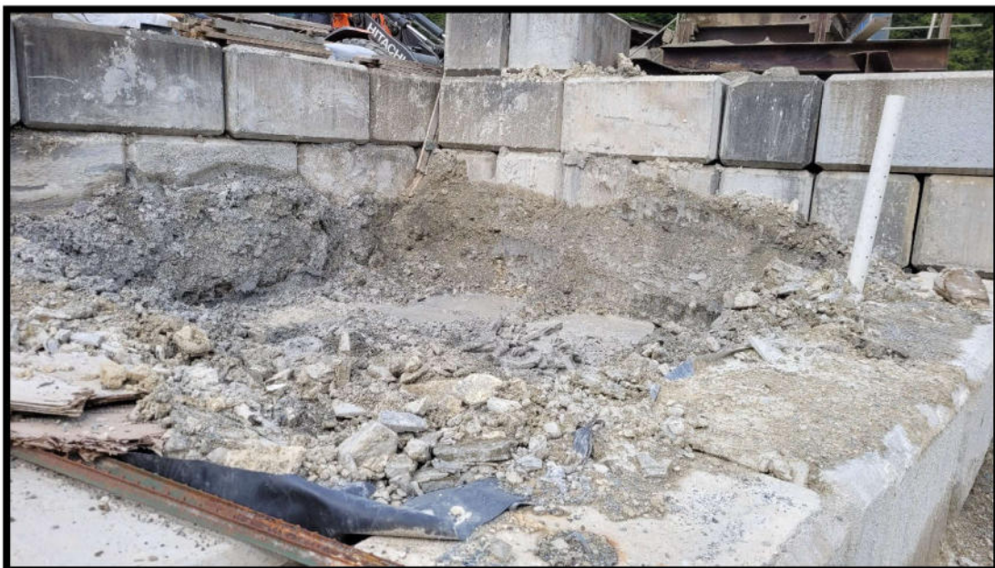
Photo 12 – Excess concrete from cleaning of drums. Recommended to maintain minimum volume in this cell to avoid overflow / flooding.
