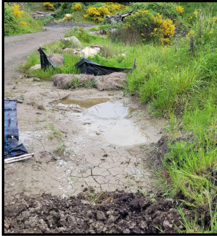
Photo 11 – Sediment buildup adjacent to silt fencing up-gradient of settling pond. It is recommended that ditching is excavated on a regular basis to avoid over sedimentation and rerouting of surface runoff.
