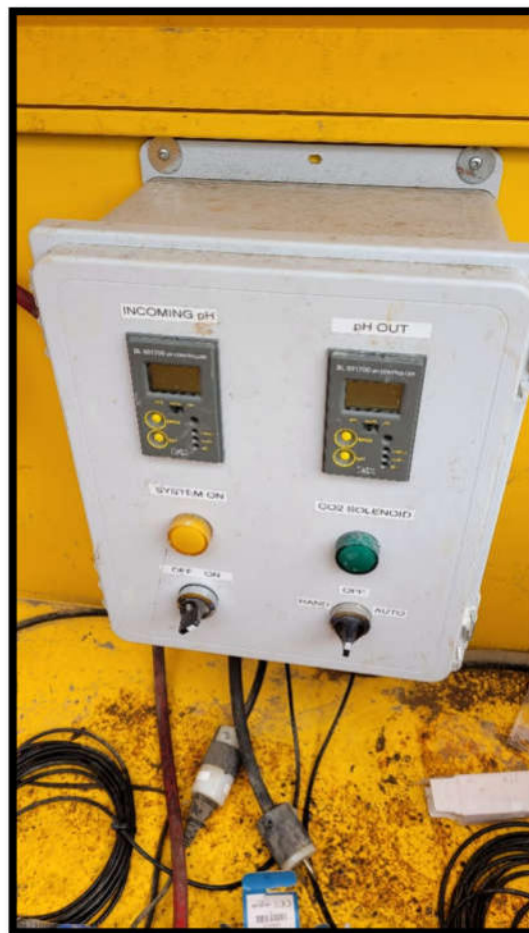
Photo 10 – Automated pH treatment controller.
