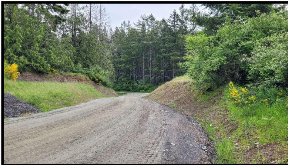
Photo 2 – Site Access ‘A’, complete with roadside ditching, gravel surfacing and stabilized banks.
