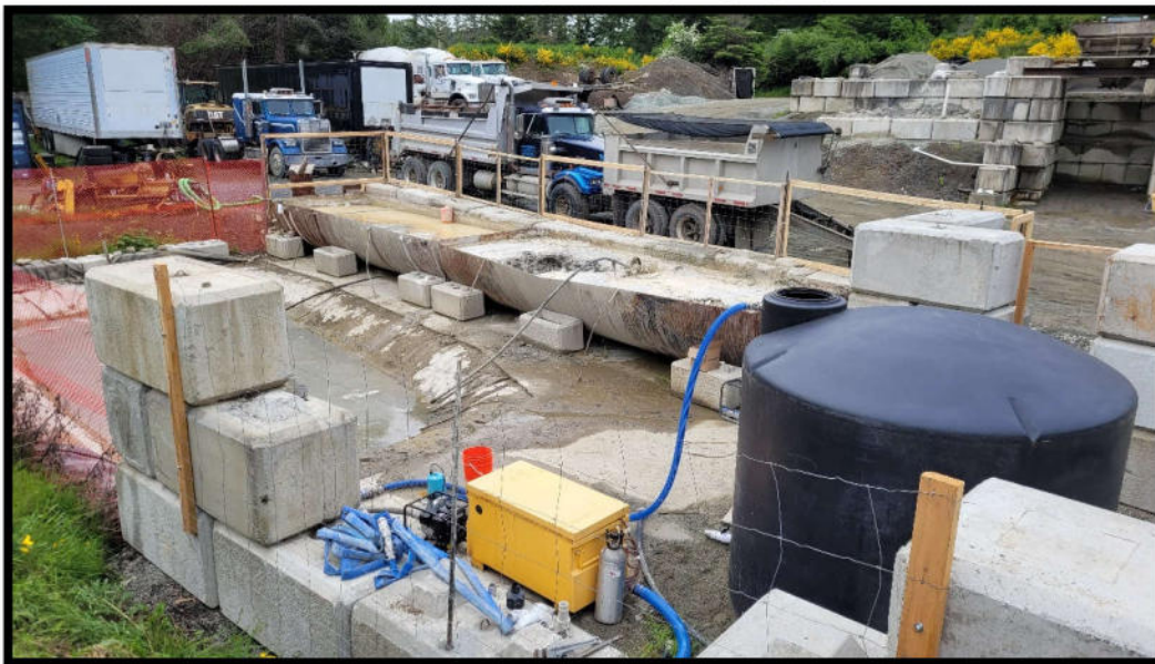
Photo 16 – Water treatment area overview.
