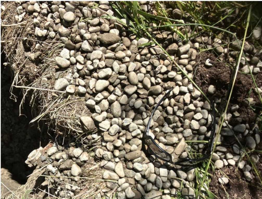
Photo 6. Gravel with sand material for backfill around slotted section of well casing, June 30, 2025.
