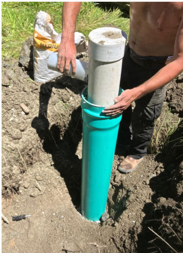
Photo 7. Pouring bentonite pellets between 6 inch diameter well casing and temporary 8 inch diameter surface casing, June 30, 2025.
