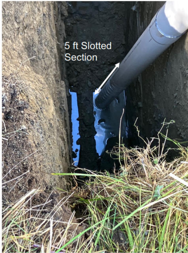
Photo 5. Monitor well casing set in excavation. Note water in bottom of excavation, June 30, 2025.
