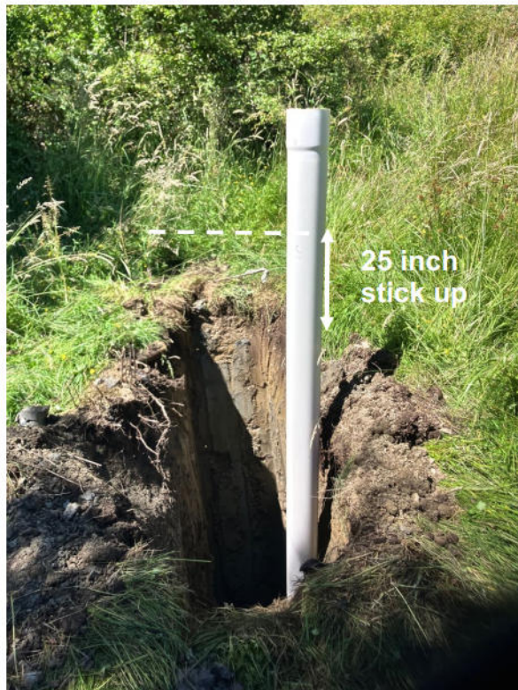
Photo 4. 6 inch diameter PVC well casing set in excavation to depth of 15 feet (4.6 m), June 30, 2025. Casing was subsequently cut to provide a 25 inch (63.5 cm) stick up above ground level.
