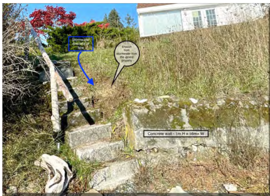
Photo #16. Stormwater direction of flow, evidence of water rills and erosion, concrete wall cracked along bottom of wall. Photo - D. Fenton. Aug 22, 2023.
