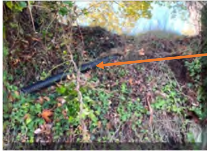
Photo #6: Big-O perforated flexible pipe to beach, end is behind a boulder. Photo credits to D. Fenton. Oct 26, 2023.
