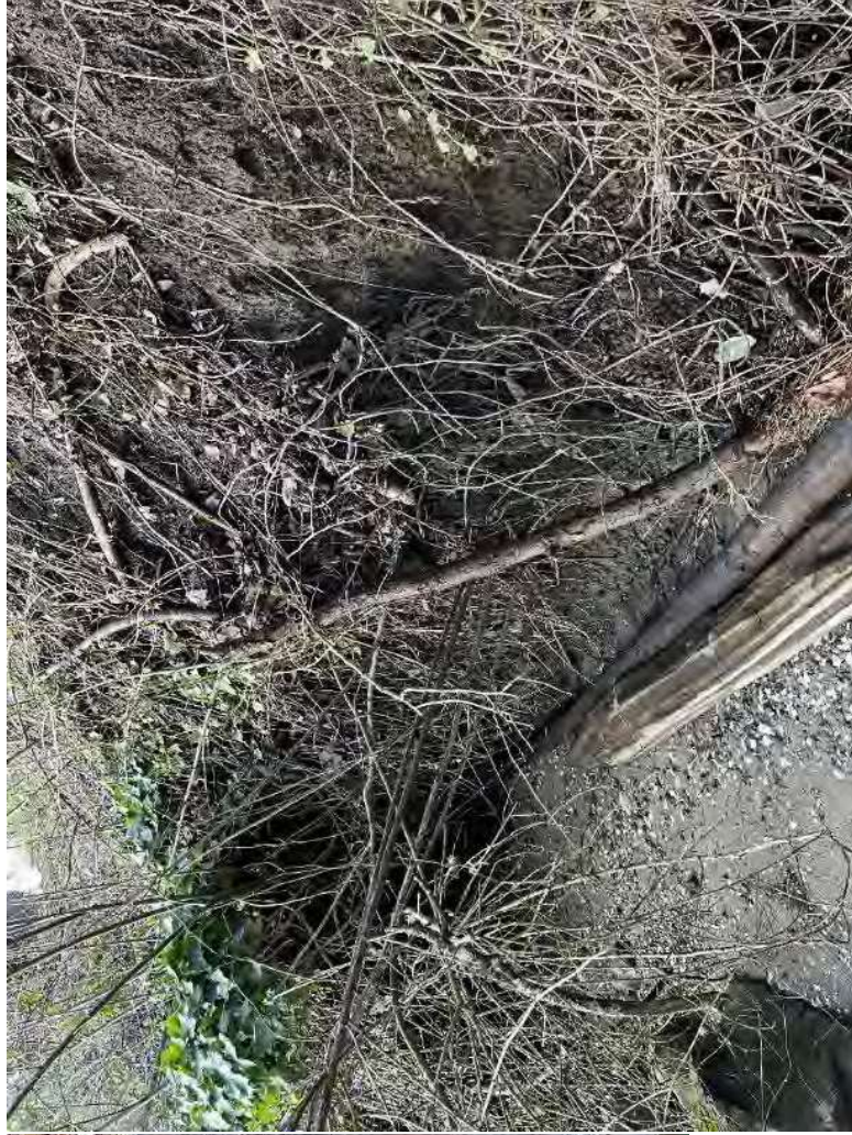
Photo 2.10 Erosion of the low coastal bluff. The bluff consists of fine silty sand material based on visual observations.
