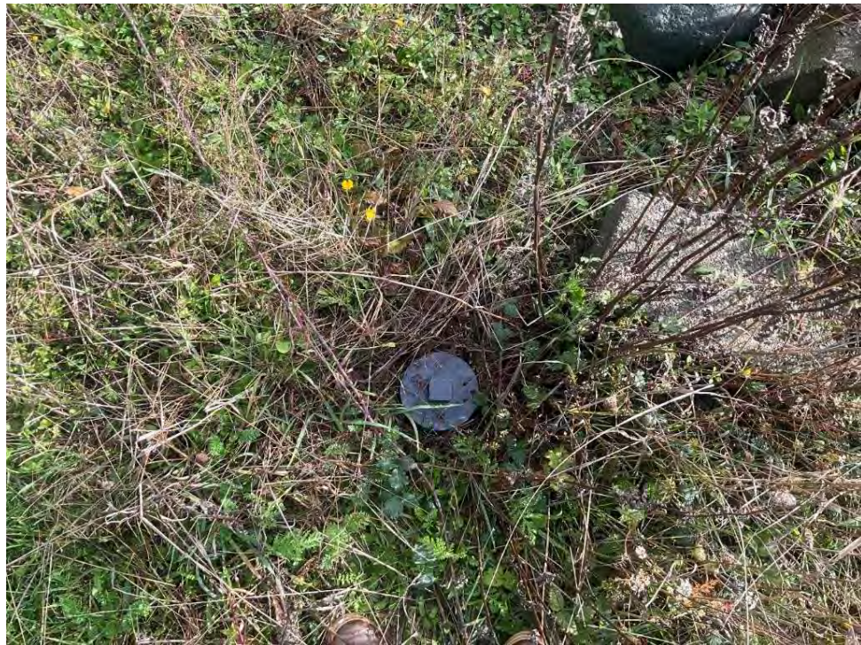
Photo 10. An ABS connection at the septic system located in the north-west of the subject lot. Potentially a connection for an adjacent pad that appeared to have an RV historically parked.
