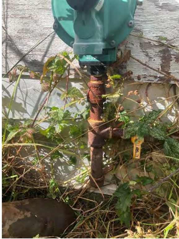
Photo 3. Disconnected propane AST connection on first residential building at the north-west of the property.
