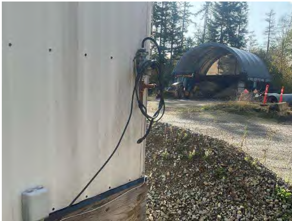
Photo 4. Disconnected propane AST connection on second residential building at the north-west of the property.
