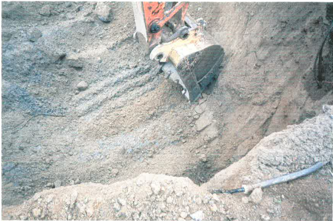
PHOTO 3: Excavation of hydrocarbon-impacted soils from former UST nest. Note dark grey hydrocarbon stained tank nest sands.
