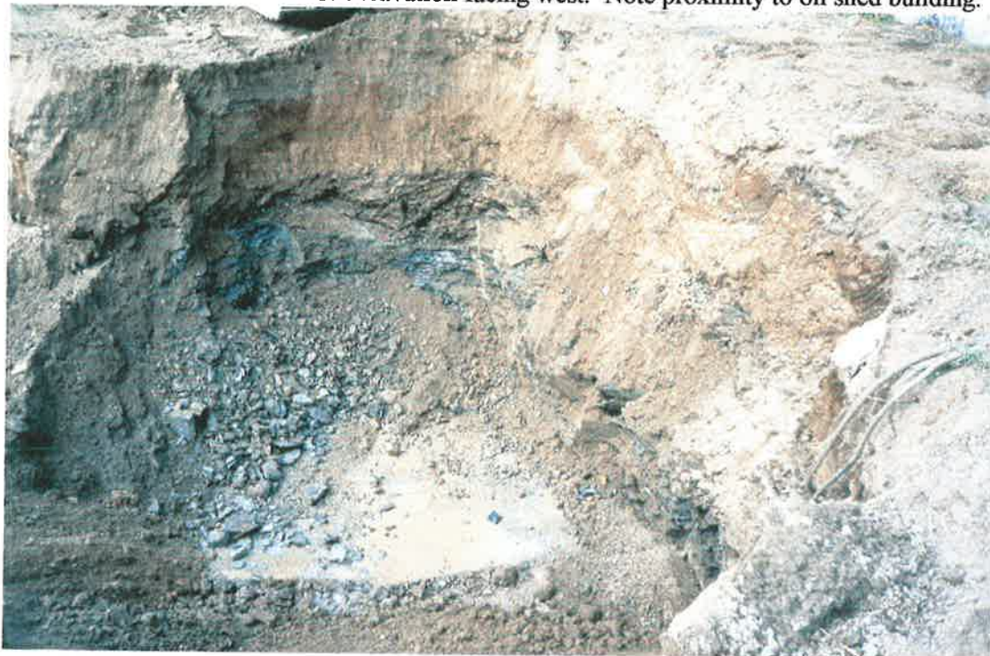
PHOTO 6: Tank nest excavation facing southwest. Note dark grey hydrocarbon-stained siltstone underlying sand and gravel fill.
