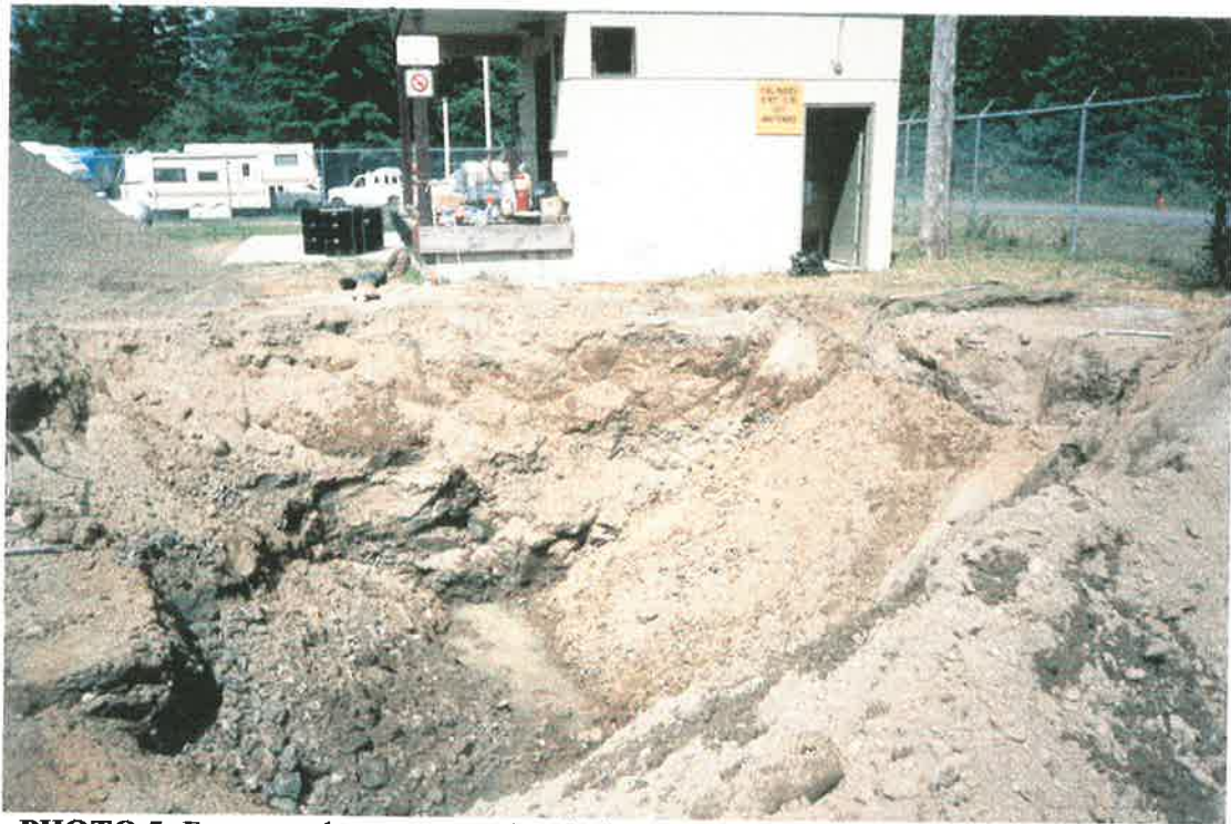
PHOTO 5: Former tank nest excavation facing west. Note proximity to oil shed building.
