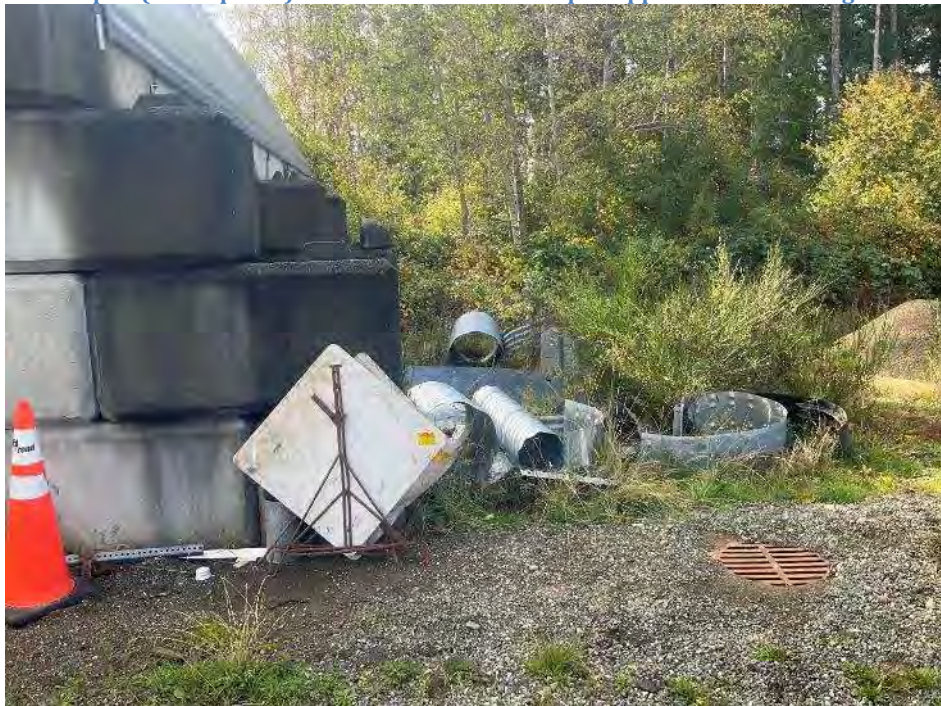
Photo 6. A manhole and catch basin located west of the salt storage shed, at a lower elevation. Presumably this feature was installed to intercept rainwater run off from the chemical storage shed.
