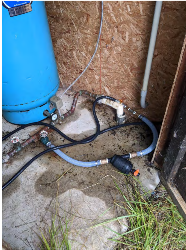
Photo 3. Pressure tank in pump house on Emcon's 3361 Piercy Road property
