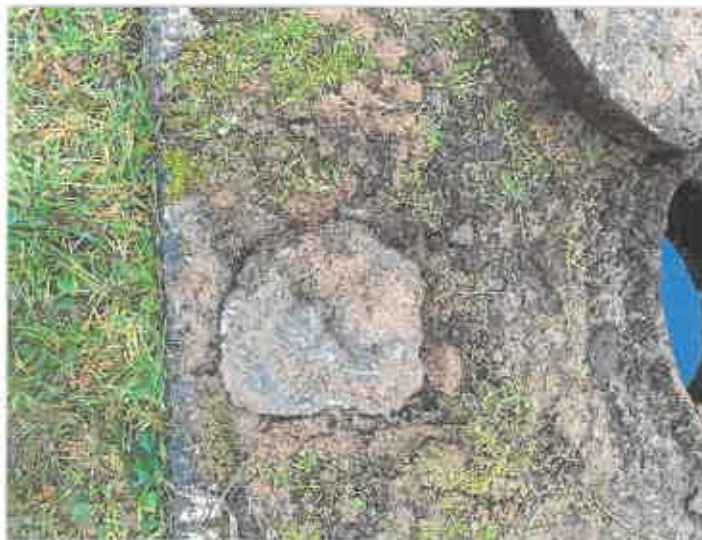
Picture 9: Inlet maintenance hatch access
