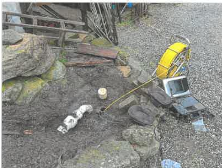
Picture 3: Limited access to interior of lift station (camera used for viewing)
