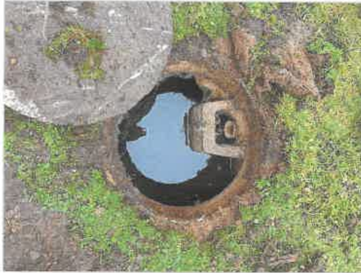
Picture 11: Location of distribution box (d-box)
