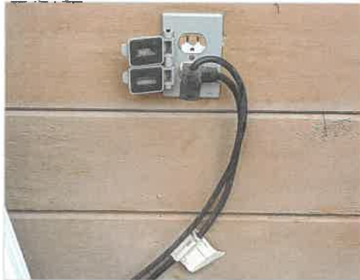
Picture 5: Electrical for pump
