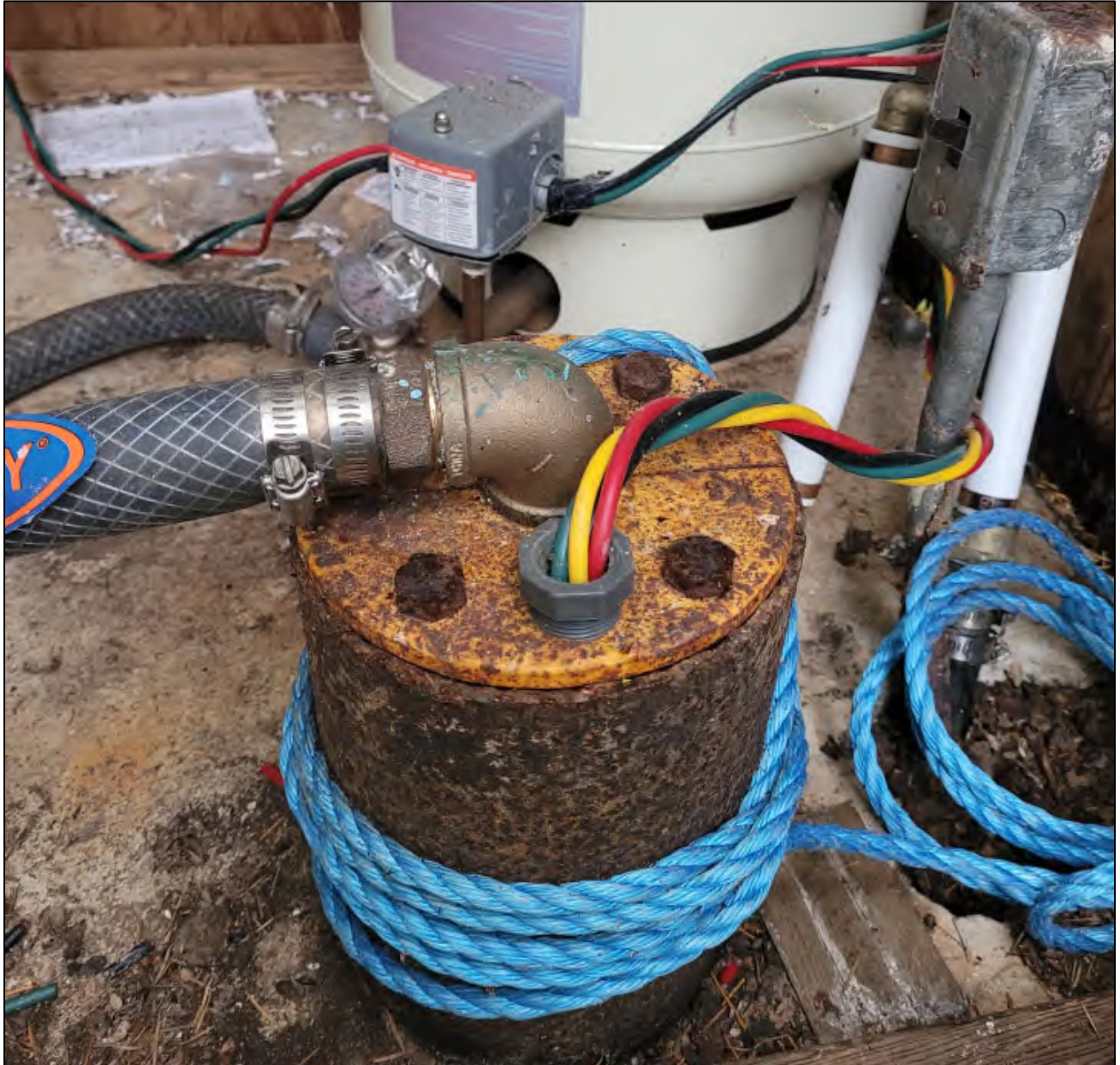
Photograph B5: Close up of the WTN 26180 wellhead. The wellhead cap could not be lifted without removing the pump, which would require assistance from a pump installer.
