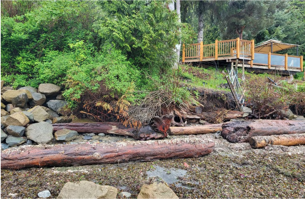
Photo 1: Western foreshore conditions where they meet neighboring revetment.
