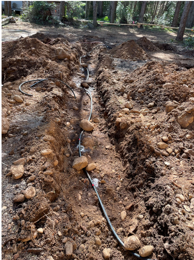
Photo. 3 Test trench dug in area of proposed wastewater dispersal field. The pipe with emitters had been discharging water for over 24 hours at a rate of about 750 Litres per day
