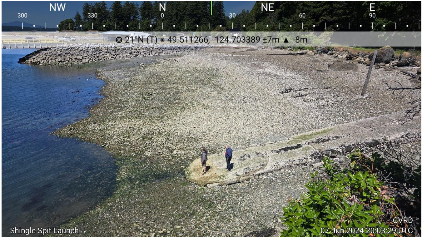
Photo 1. Showing the current condition of the boat launch as viewed from the adjacent breakwater. Note the BC ferries dock in the background. The new launch will extend seven meters from the end of the existing dock into the shallow area visible at bottom left of photo. The people in the photo were hoping to launch a small boat at the time of the assessment but the tide was too low to allow for a safe launch.
