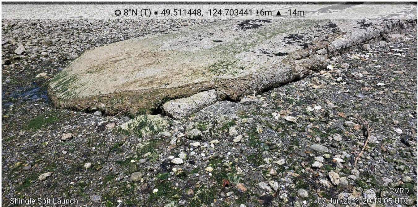
Photo 2. Showing the current condition of the boat launch, note eroded end of the launch.
