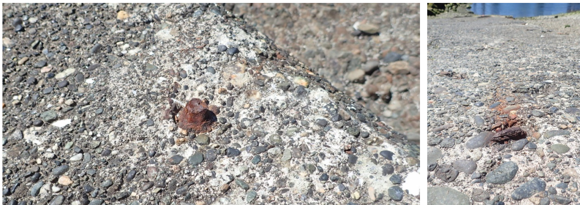
Figure 5 – Rebar Out of Surface
