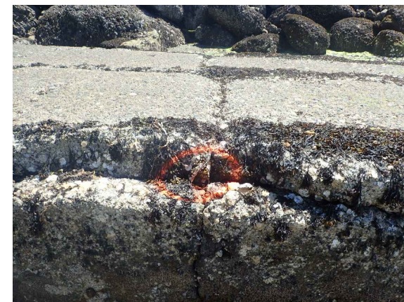
SEVERE OVERSTRESSING ON TOP SLAB OF RAMP
