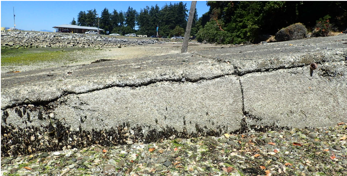
Figure 8 – Longitudinal and Vertical Cracks
