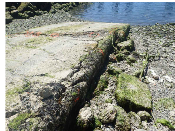
LOWER RAMP WITH SEVERE DETERIORATION TO CONCRETE
