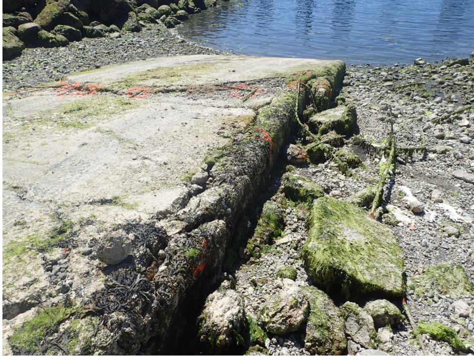
Figure 10 – View of Lower Ramp Spalled Concrete and Reinforcement
