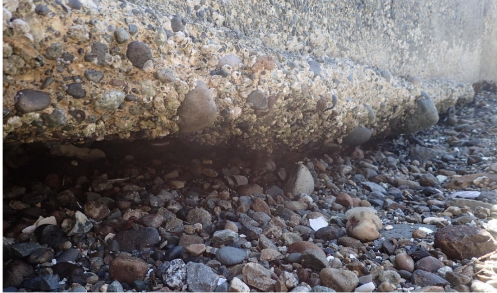
Figure 11 – View of Gap Beneath Wall
