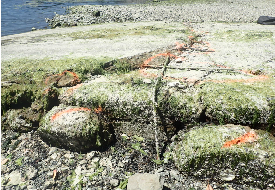
Figure 6 – Bottom End Exposed Rebar and Loose Concrete
