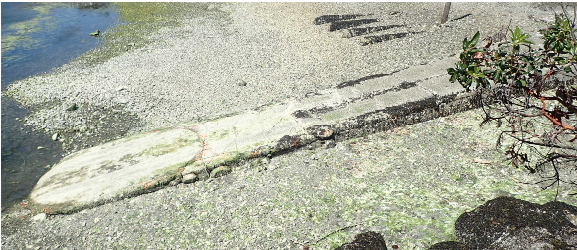
Figure 4 – View of Lower Ramp with Water Damage
