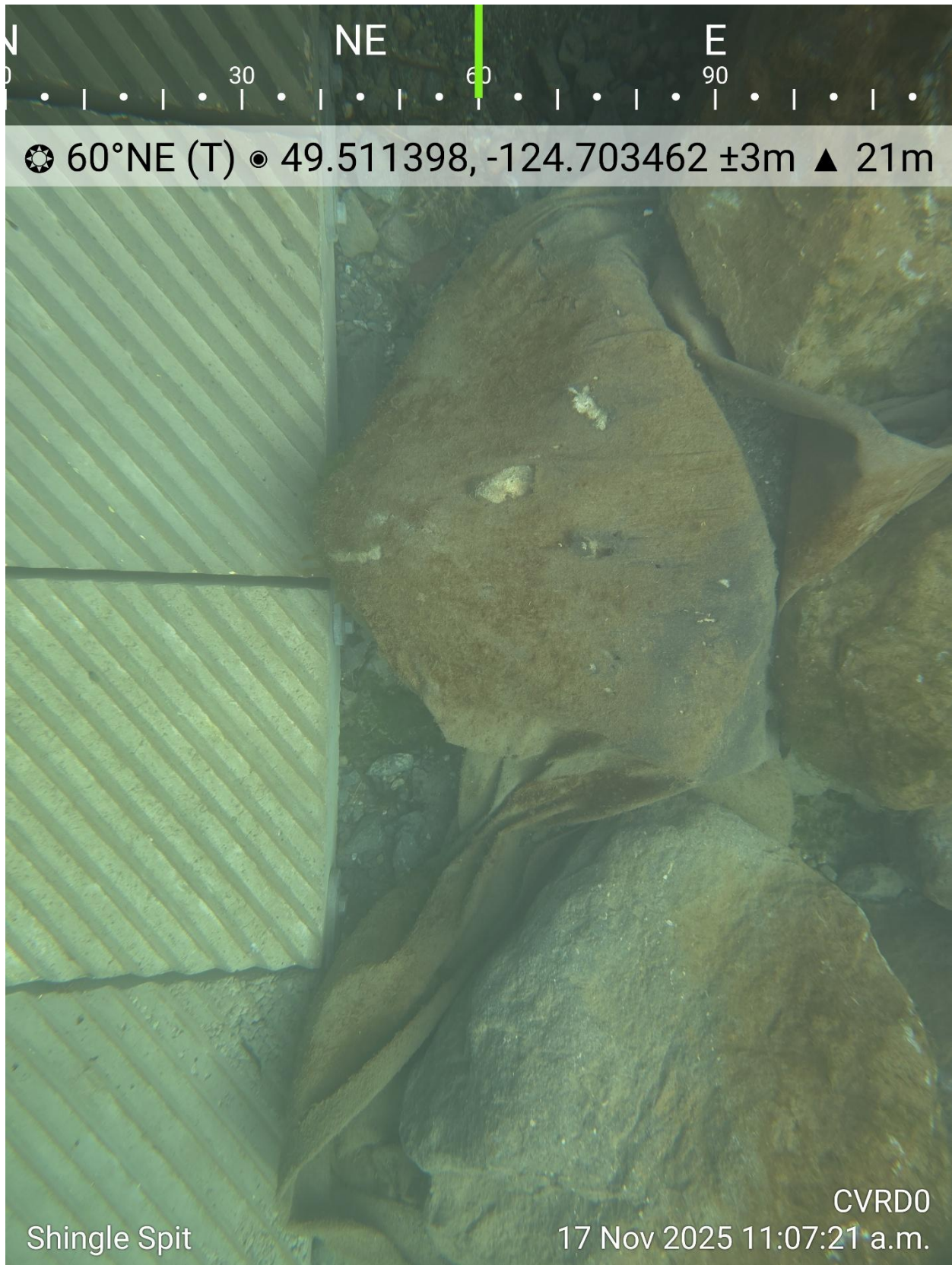
Photo 2. Showing excess geotextile cloth along the riprap on the north side of the ramp, below the water line during the 17-Nov.-2025 site inspection.
