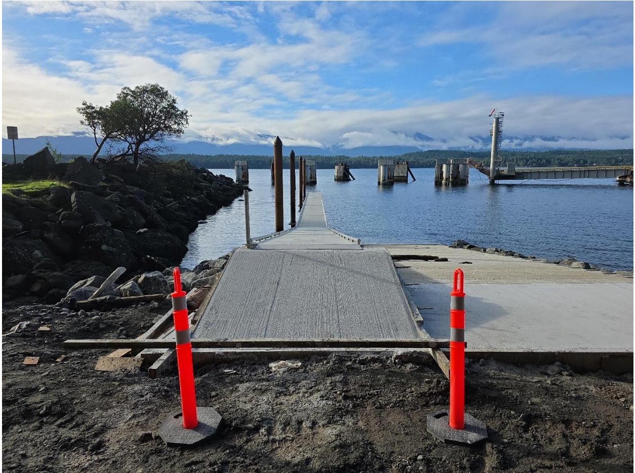
Photo 7. Showing recently cured concrete at the top of the ramp as well as the transition area that needs to be filled in.
