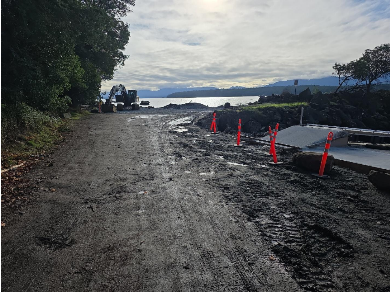
Photo 6. Showing muddy areas and minor water pooling on the driving surface that could benefit from some minor contouring. Exposed soils that remain along the foreshore (at right), should be seeded with an appropriate erosion inhibiting seed mix.
