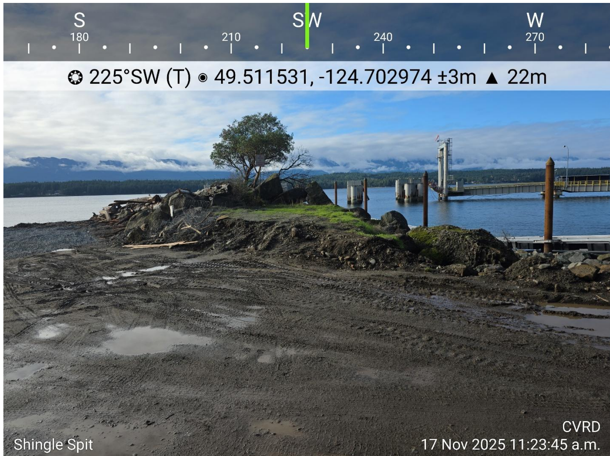
Photo 8. Showing cut-slope at the landward end of the breakwater that should be grass seeded. Also note the waste fencing at center left that should be cleaned up. The pile of beach wood behind the fencing, as well as another small pile at the south side of the parking/barge landing area, should also be distributed in a “natural” configuration across the foreshore.
