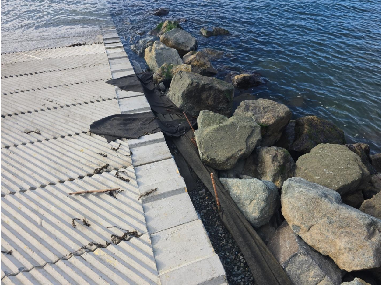
Photo 3. Showing excess geotextile cloth along the riprap on the north side of the ramp during the 17-Nov.-2025 site inspection. Note the large gap between the cloth and the edge of the ramp. Rebar shown in this photo should also be removed.
