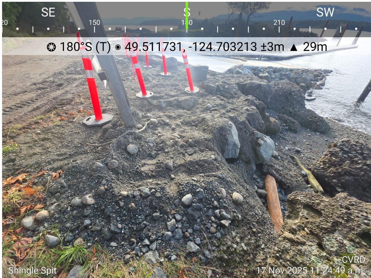
Photo 5. Fill material on the edge of the ramp should be pulled back and used to create a smooth transition from the roadway to the top of the ramp. This area, as well as any other areas of bare soil off of the driving surface, should be grass seeded.
