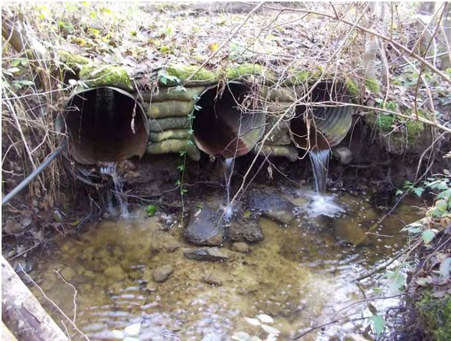
Looking upstream at the culverts that direct the stream under a residential access road.
