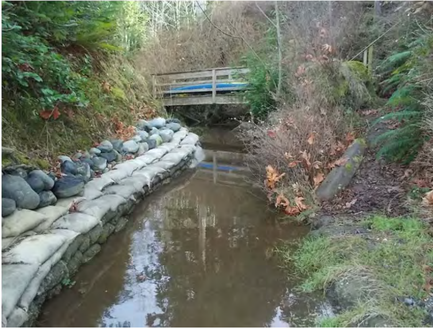
Looking southeast from the natural boundary of the marine environment. Note the placement of boulders, cement and sandbags for the purpose of stabilizing the bank.
