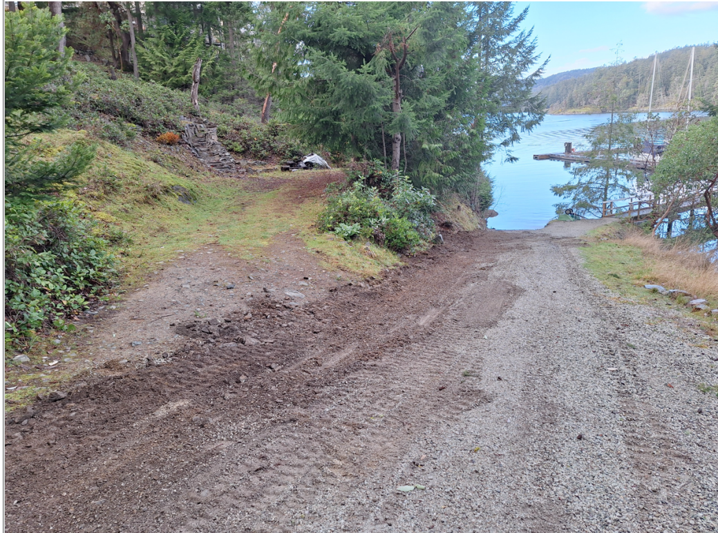
Completed installation - Trenched split pipe at the Connected Coast Musgrave Boat Ramp
