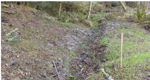
Photo 11. Habitat upstream of Northwest culvert. Property boundary at right-hand side of photo.
