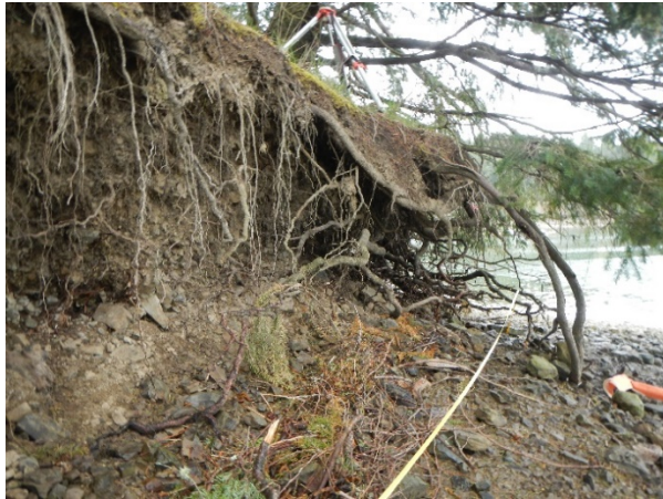
Photo 1. Steep eroding bank at the high tide line of the intertidal transect (Transect 3, Figure 2). Higher high-water swash is at the base of the bank.
