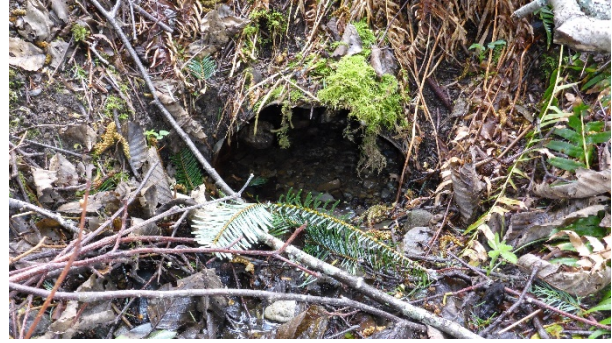
Photo 20. Outlet of South culvert. Culvert 50% blocked with debris.
