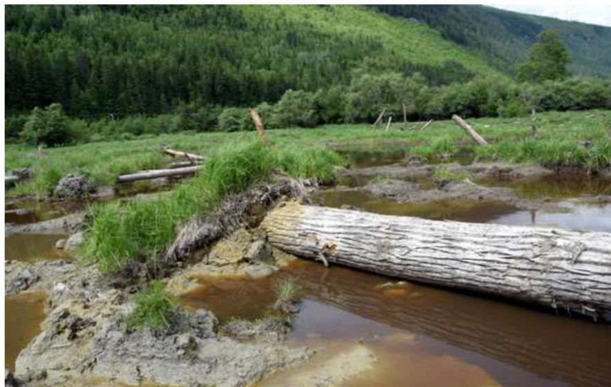
Large diameter logs would be placed in the restored wetlands to resemble trees naturally falling over. This photo shows one of many dead trees placed in wetlands restored at Meadow Creek in January 2016.
