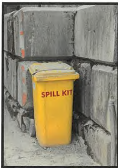
Photo 15: Spill kit located within batching area.
