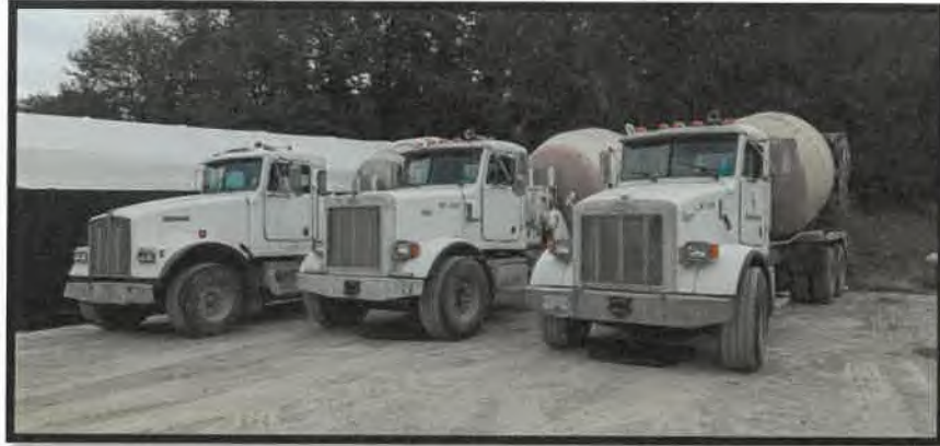
Photo 17: Drip trays noted below concrete trucks.
