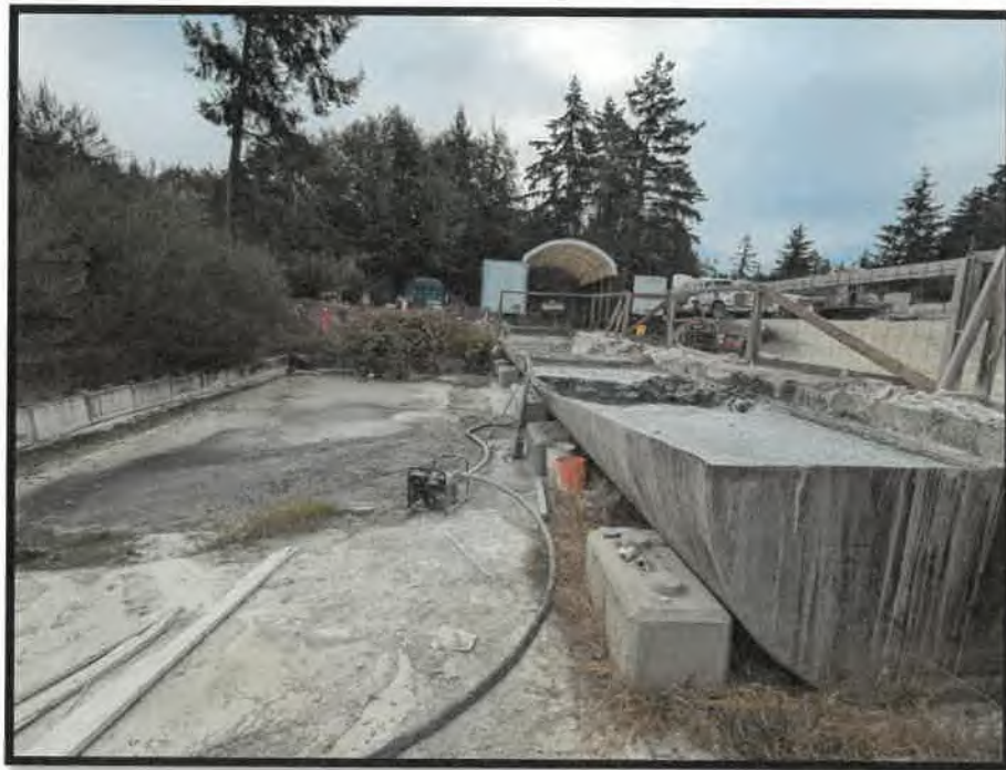
Photo 8: Water management area requires cleanout prior to rainy season.
