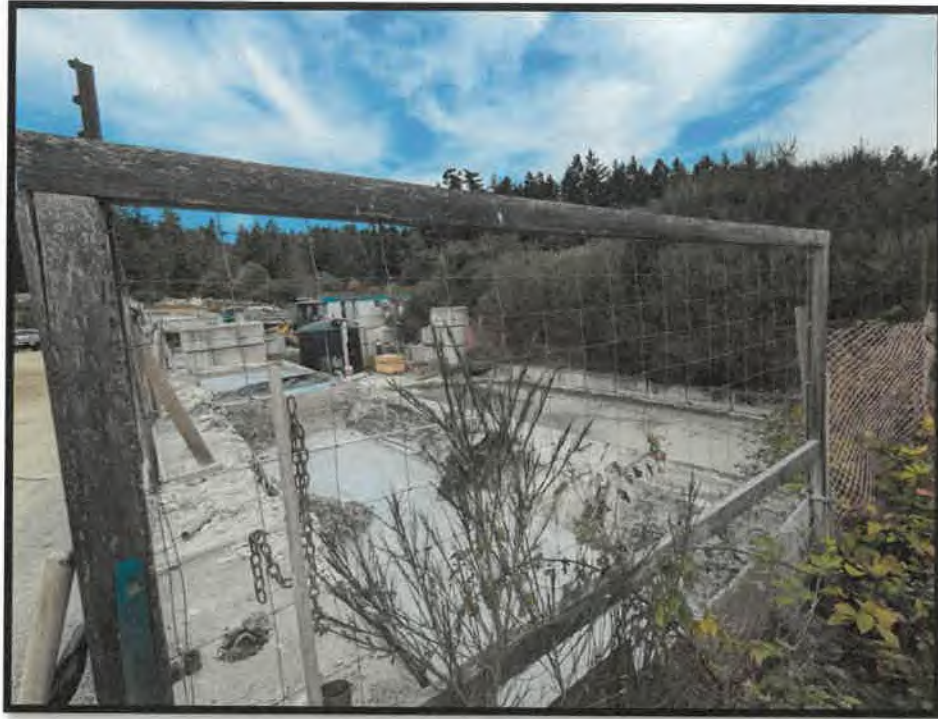
Photo 7: Water management area showing one of two holding tanks with available capacity.
