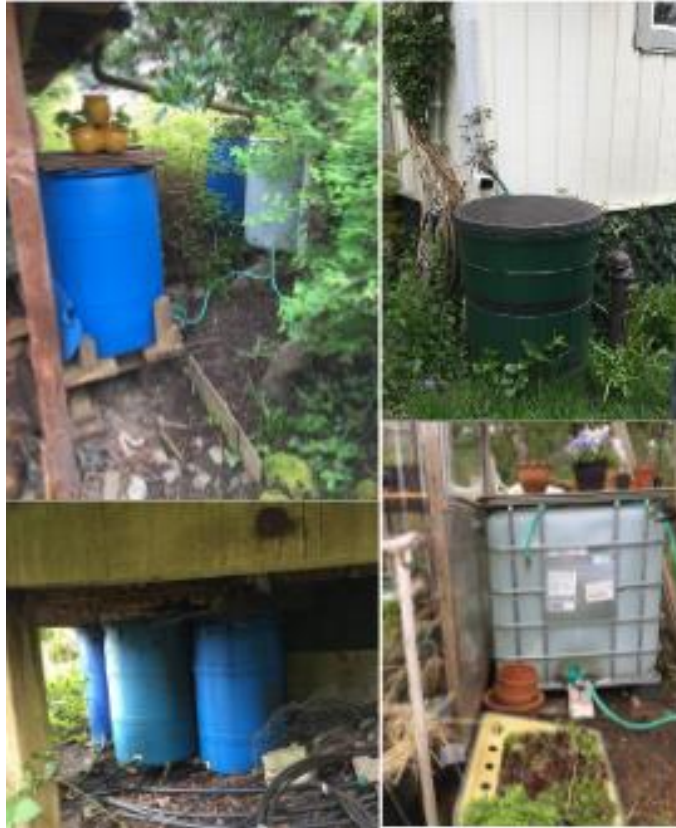
Figure D9. Case study S3 images taken by Kendra Anderson during site visit on April 23, 2017 to gather further details on RWH systems that exist on SSI. A variety of tanks are used to store rainwater, including a 1,000 liter food shipping container, for a combined 5,000 liter storage capacity.
